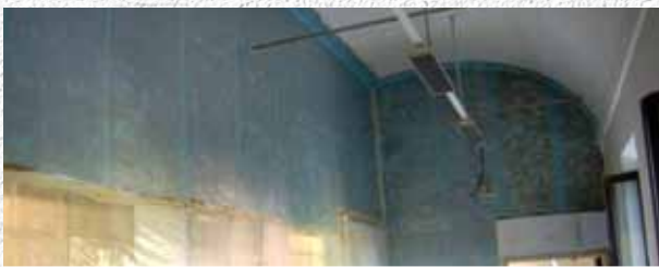
Application of MapeWrap EQ System on a wall. Pio. Middle School. Carpi, Modena, Italy.
