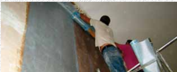
Application of MapeWrap EQ System on a wall. Pio. Middle School. Carpi, Modena, Italy.
