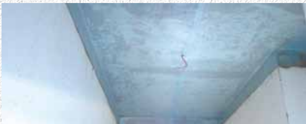
Application of MapeWrap EQ System on a ceiling. Private house. Finale Emilia, Modena, Italy.
